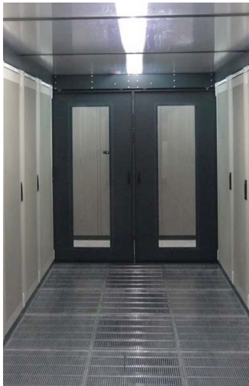
Example of a Cold Aisle Corridor
